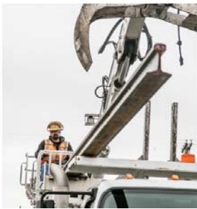
Automated Rail Unloading
