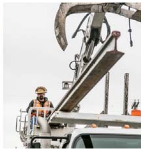
Automated Rail Unloading
