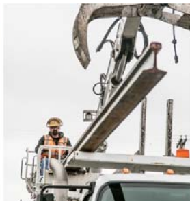
Automated Rail Unloading
